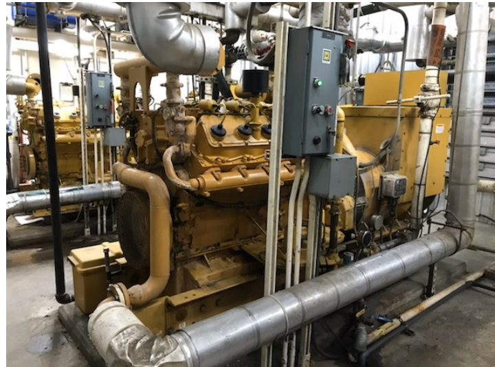
One of three 214 kW CHP generation units
