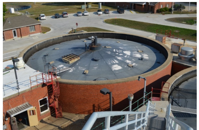
One of four anaerobic digesters, aerial view
